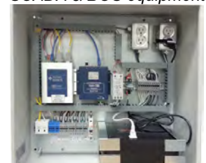
SCADA & BOS equipment
